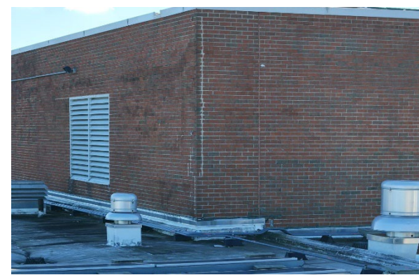
Image 2.27: P5- Repointing and Concrete Cap Repointing of mortar joints at existing brick wall and repair of deteriorated concrete cap is required.
