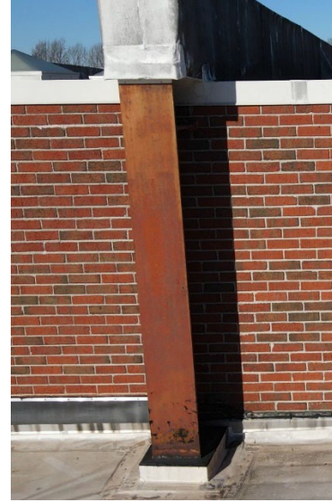
Image 2.38: P16- Exposed Column
