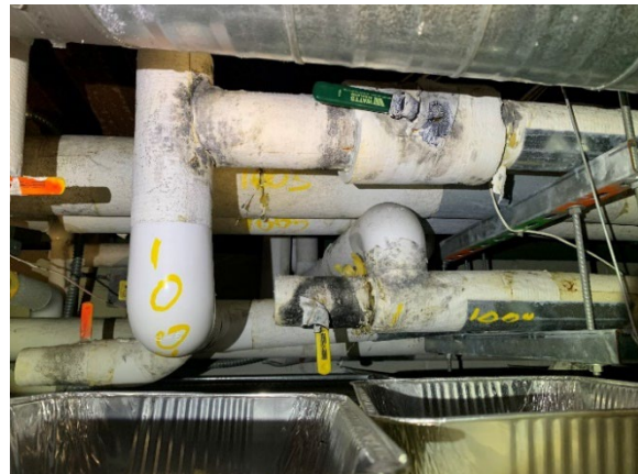
Image 4.6: Improper Insulated Pipe
