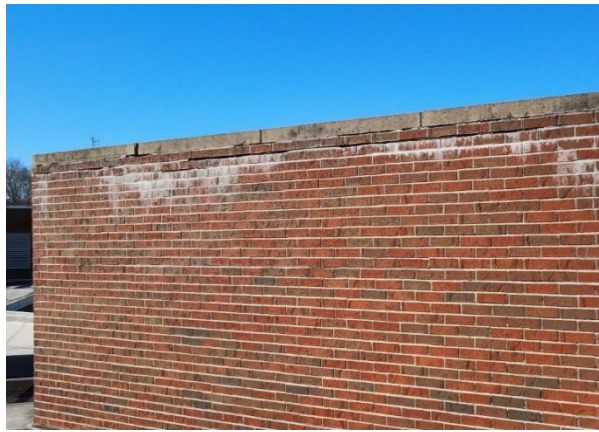
Image 2.25: P3- Repointing and Concrete Cap Repointing of mortar joints at existing brick wall and repair of deteriorated concrete cap is required.
