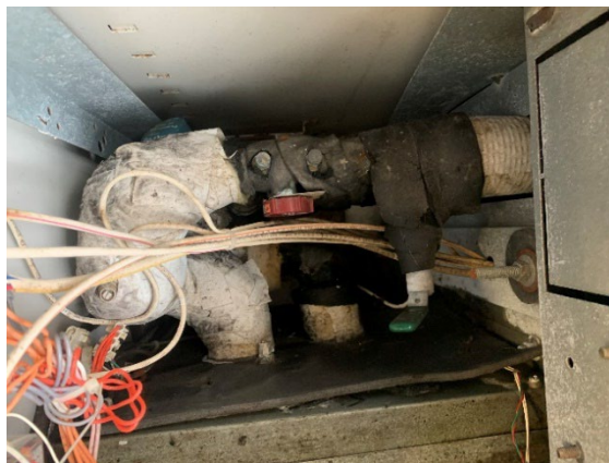
Image 4.11: Typ. Unit Ventilator Piping
