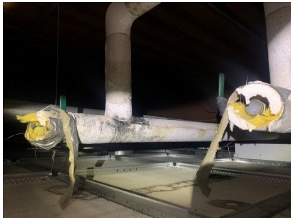
Image 4.5: Improper Insulated Pipe
