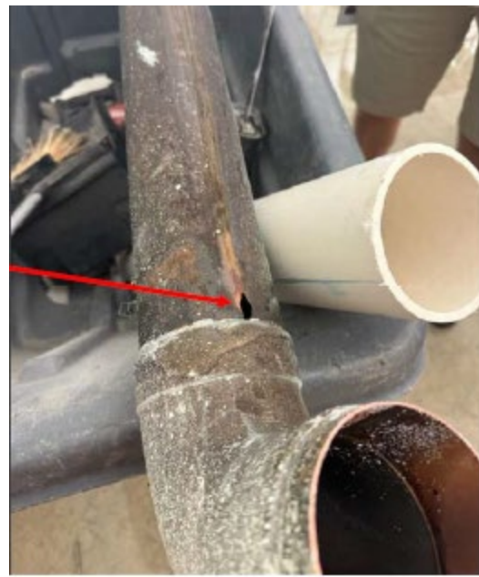
Image 3.2: Hole in Existing Roof Drain Line
