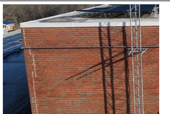
Image 2.30: P8 – Repointing of Mortar Joints Some bricks have cracks through them, which were patched. Cracked bricks need to be replaced with new bricks.
