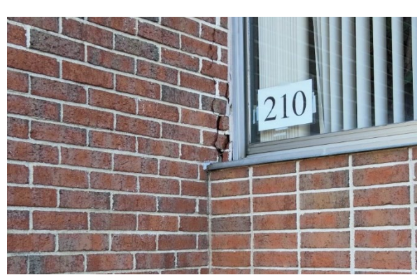
Image 2.28: P6 – Repointing of Mortar Joints Re-pointing of mortar joints at existing brick wall.
