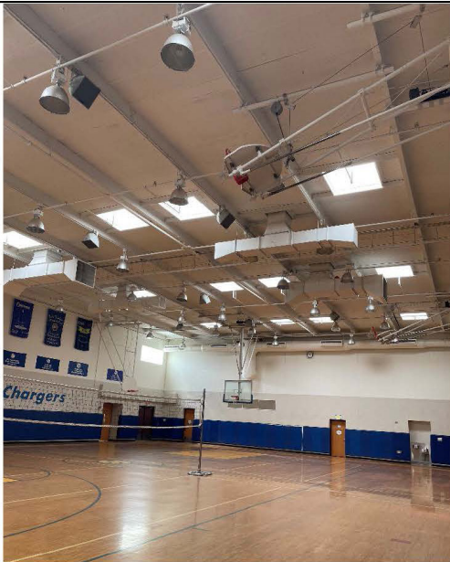
Photo # 47: - Gymnasium High Bay Lights
