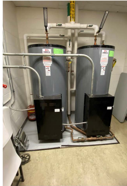
Photo # 14: Existing electric domestic water heaters.
