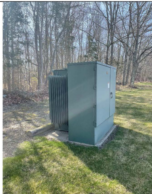
Photo # 27: - Utility Pad Mounted Transformer
