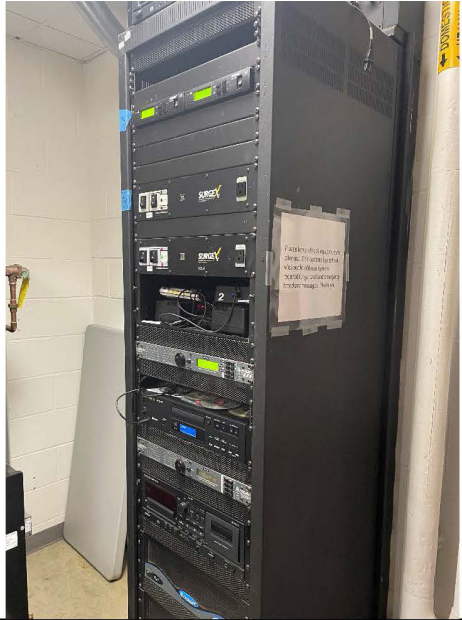
Photo # 57: - Audio System Rack
