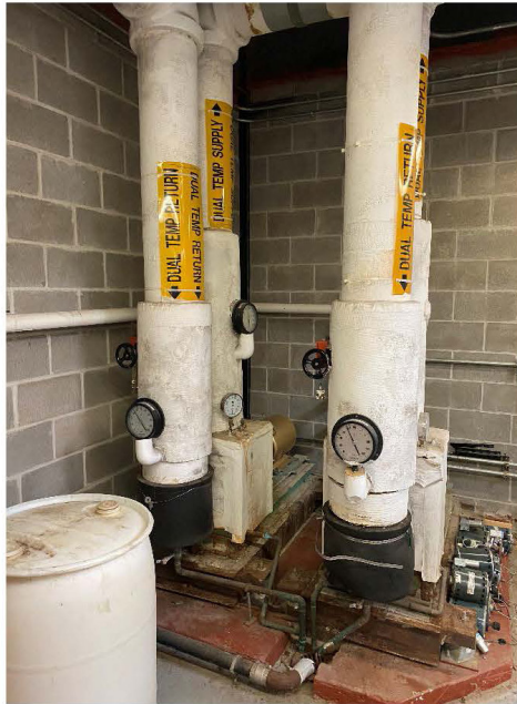
Photo # 5: Dual temp base mounted pumps.
