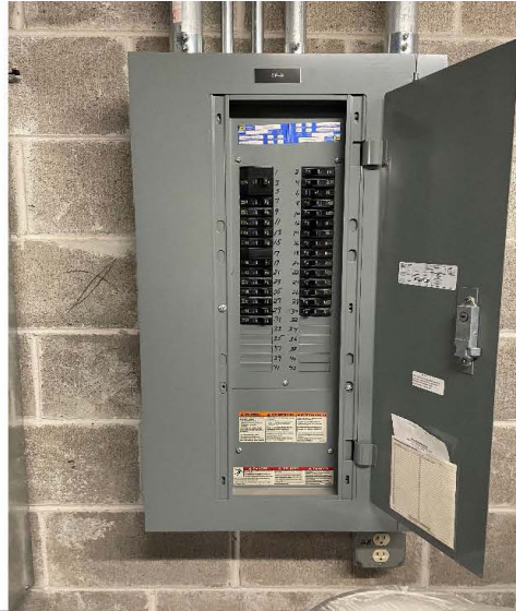
Photo # 30: - Typical "CP" for Mechanical Equipment
