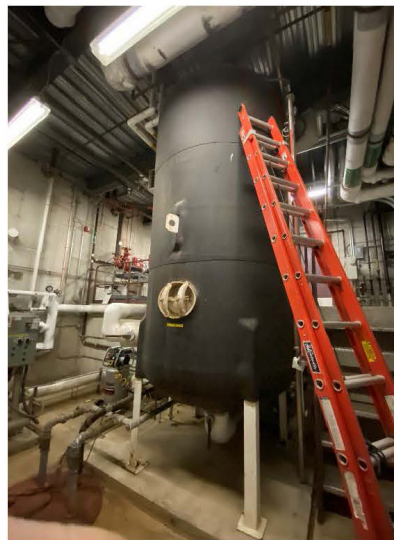
Photo # 8: Water storage tank.
