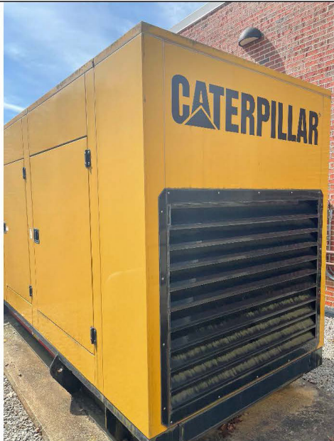
Photo # 37: - 400kW/500kVA Diesel Powered Generator with Sub-Base Fuel Tank
