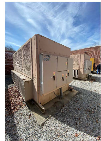
Photo # 12: Existing air cooled chillers.
