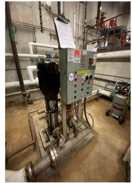
Photo # 10: Domestic water booster pump system.
