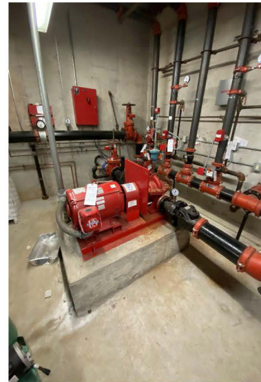
Photo # 11: Fire pump and sprinkler riser assembly.
