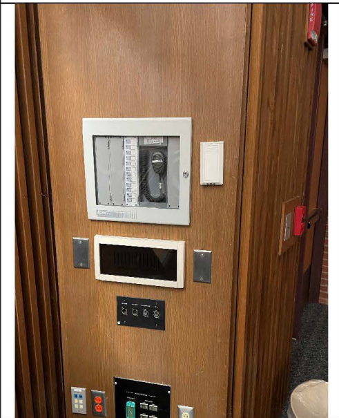
Photo # 52: - Fire Alarm Voice Evac Panel in Auditorium
