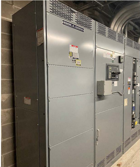
Photo # 29: - Service Entrance Switchboard in Main Electric Room
