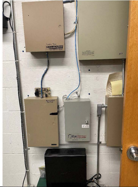
Photo # 58: - Access Control System Headend Equipment
