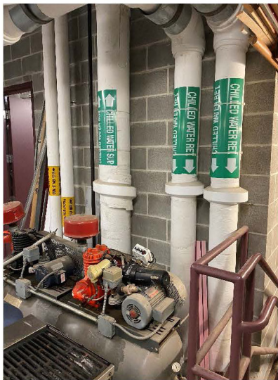
Photo # 7: Chilled water distribution piping.
