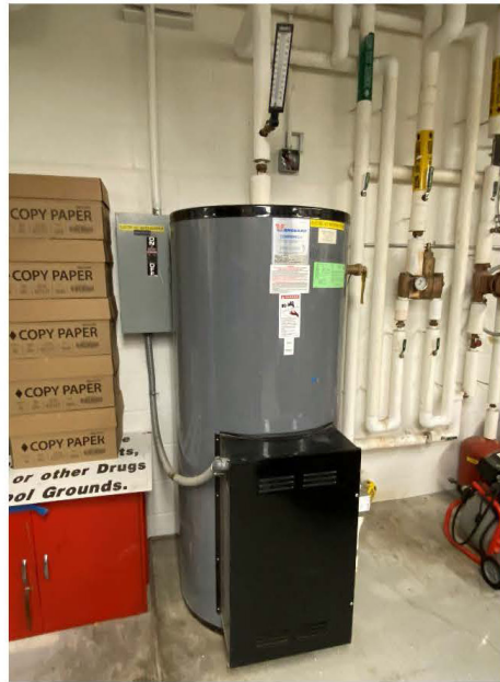
Photo # 1: Electric water heater with mixing valves.
