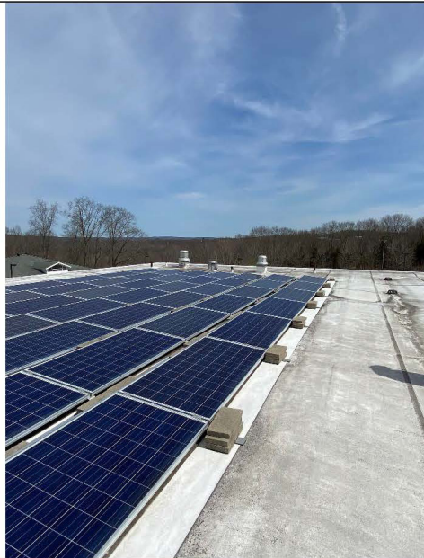
Photo # 38: - Solar Panels on Roof
