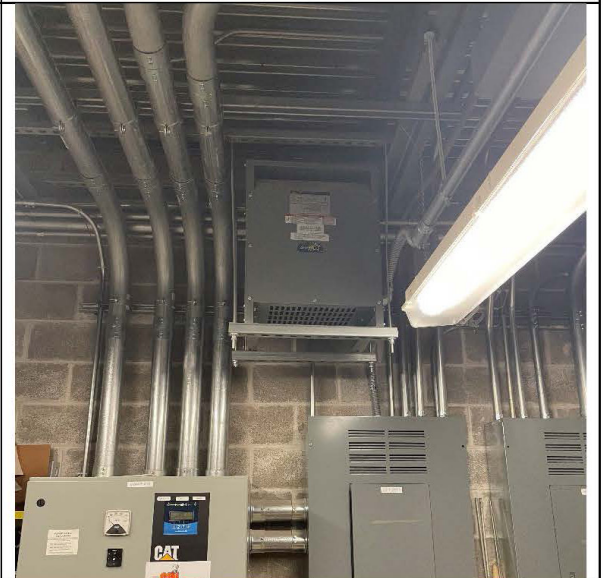
Photo # 36: - Standby ATS with Distribution Panel “ESB-1” and Transformer for Panel “EOP”
