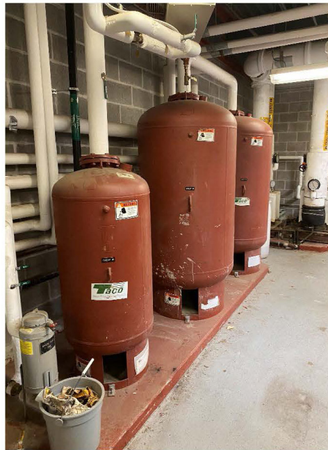
Photo # 6: Expansion tanks for hydronic systems.
