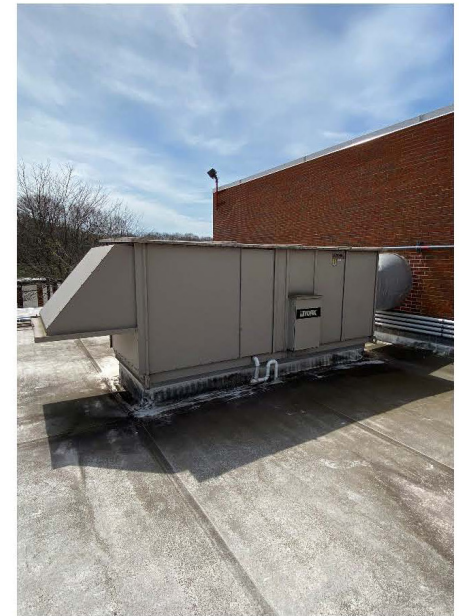
Photo # 18: Existing air handling unit.
