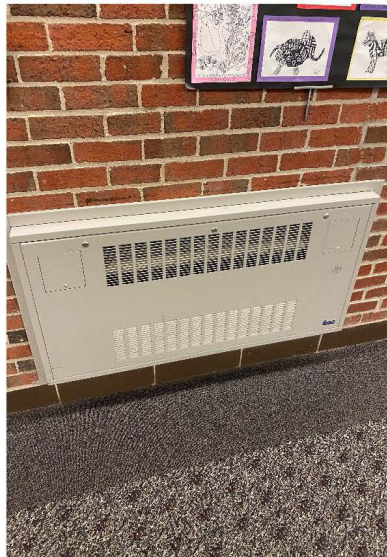
Photo # 15: Semi recessed cabinet unit heater.
