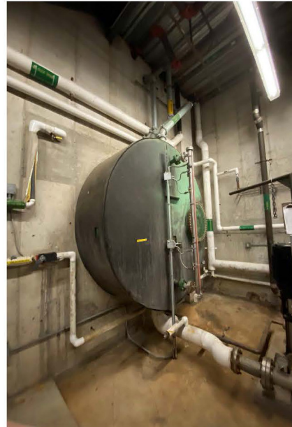
Photo # 9: Buried water storage tank.
