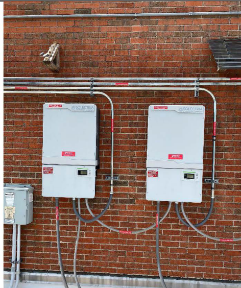
Photo # 40: - Typical Photovoltaic System Inverters on Roof
