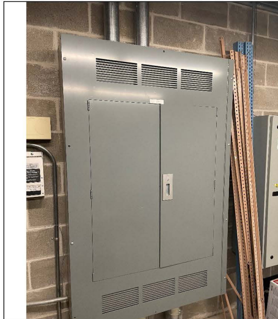
Photo # 33: - Emergency Distribution Panel “EDP”
