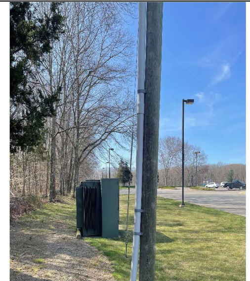
Photo # 26: - Utility Service Pole Primary and Telecommunications with Utility Transformer
