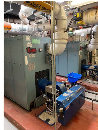
Photo # 4: Existing boiler plant.
