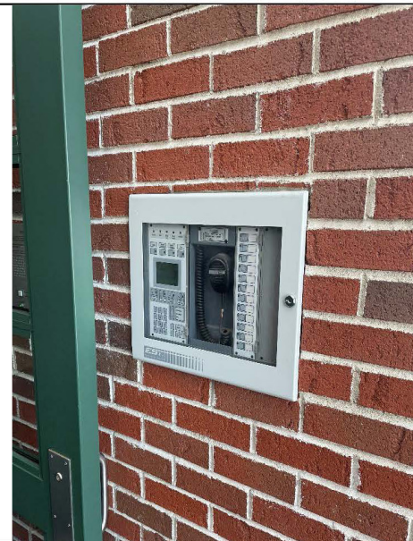
Photo # 51: - Fire Alarm Remote Annunciator Panel in Main Entrance Vestibule
