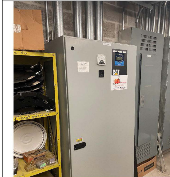
Photo # 35: - Automatic Transfer Switch – 600A (Optional Standby)
