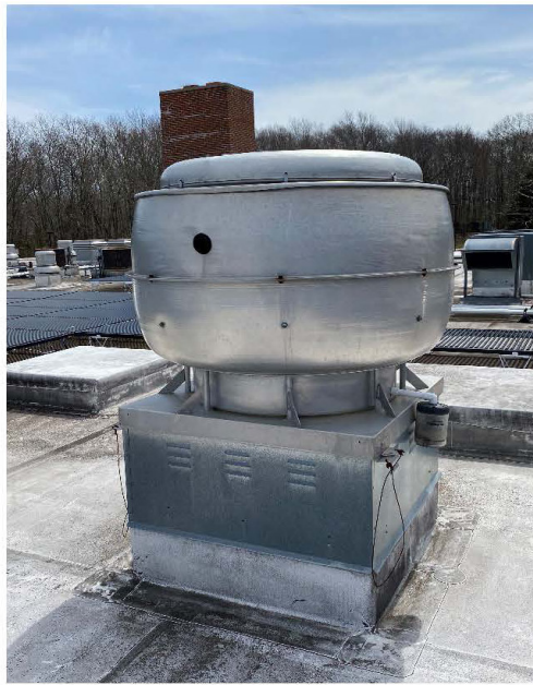
Photo # 22: Kitchen exhaust fan
