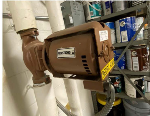
Photo # 3: Domestic hot water re-circulation pump.
