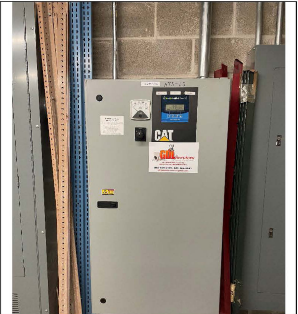
Photo # 34: - Automatic Transfer Switch – 150A “ATS-LS” (Life Safety)
