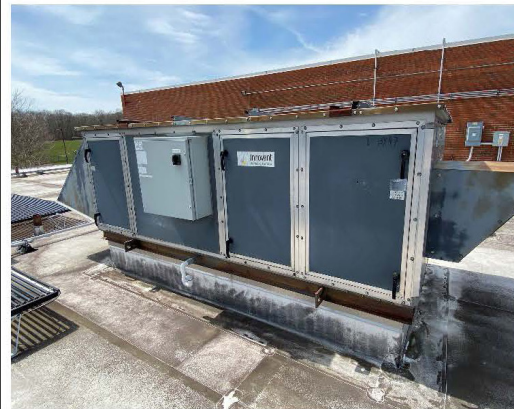
Photo # 19: Gas fired heat pumps- installed in 2017.
