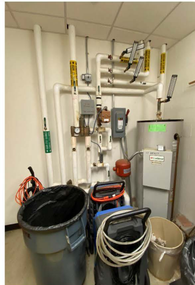
Photo # 16: Additional electric water heater in storage room.
