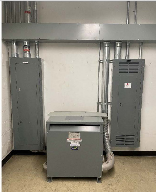
Photo # 31: - Typical Electrical Closet Panels and Distribution Transformer
