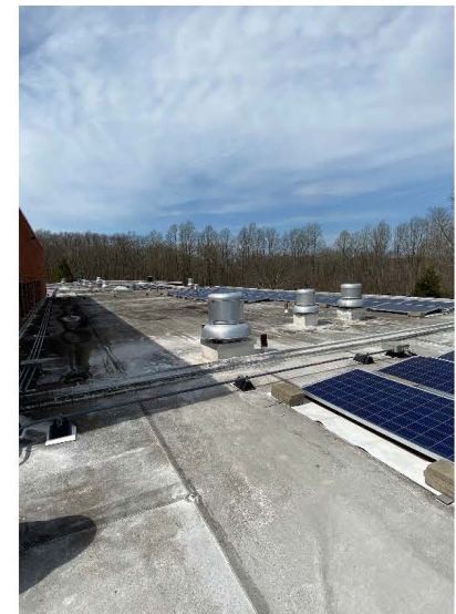
Photo # 20: Typical roof mounted exhaust fans.
