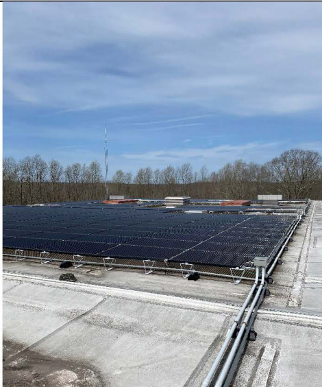
Photo # 39: - Solar Panels on Roof
